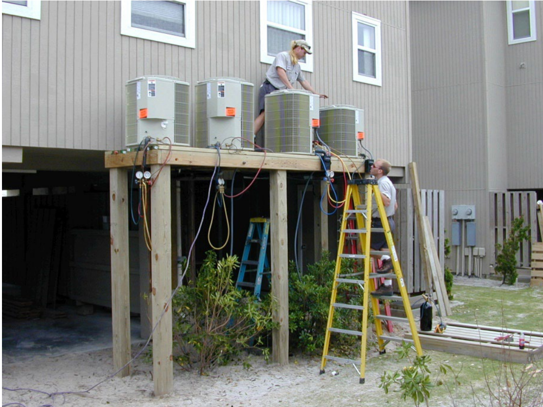
Figure 11: Elevating mechanical equipment in Carolina Beach, NC to protect against coastal flooding.
