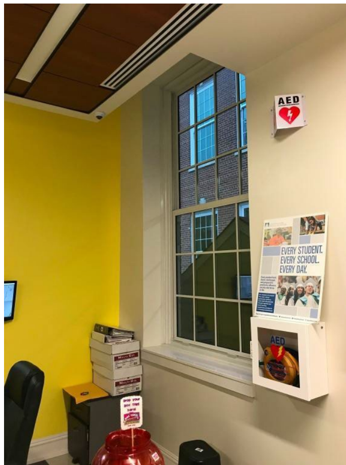
Figure 19: A dropped ceiling at the Capitol Hill Montessori School near Union Station, showing how daylighting is still able to enter the room. In some situations, drop ceilings from previous modernizations can be removed to allow full ceiling height to be restored, further improving daylight distribution.
