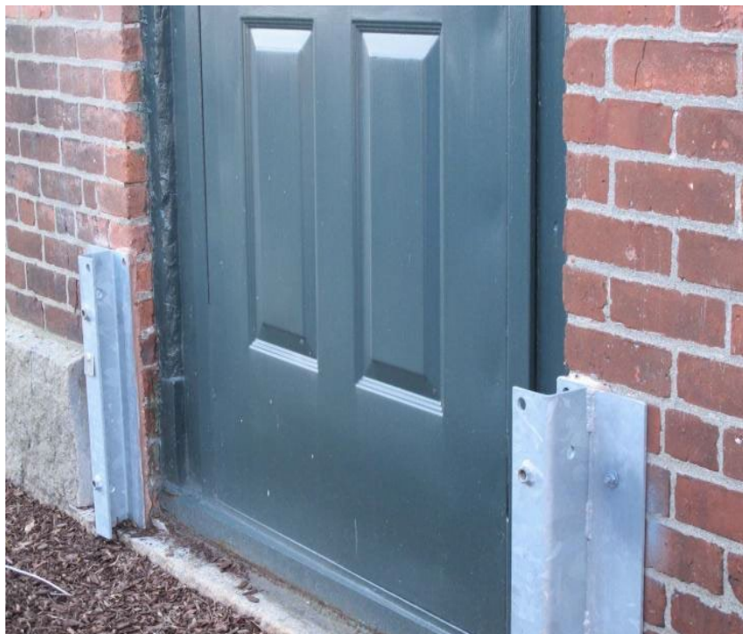
Figure 9: Track for demountable flood barrier that can be deployed in advance of a possible flood event. This retrofit of a 19th Century mill building converted into commercial office space in Providence, RI will protect against about a foot of flooding.
